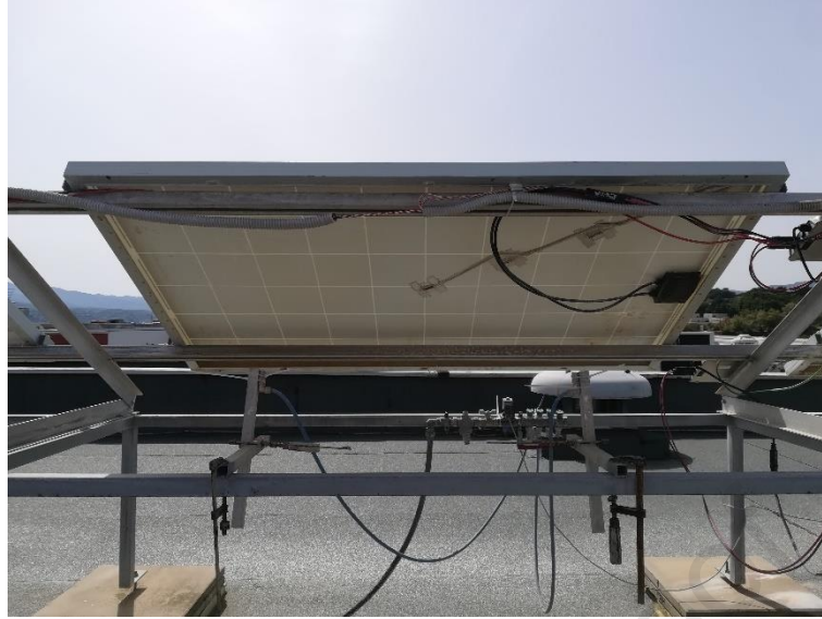
Fig. 3. PV panel equipped with spray cooling nozzles
